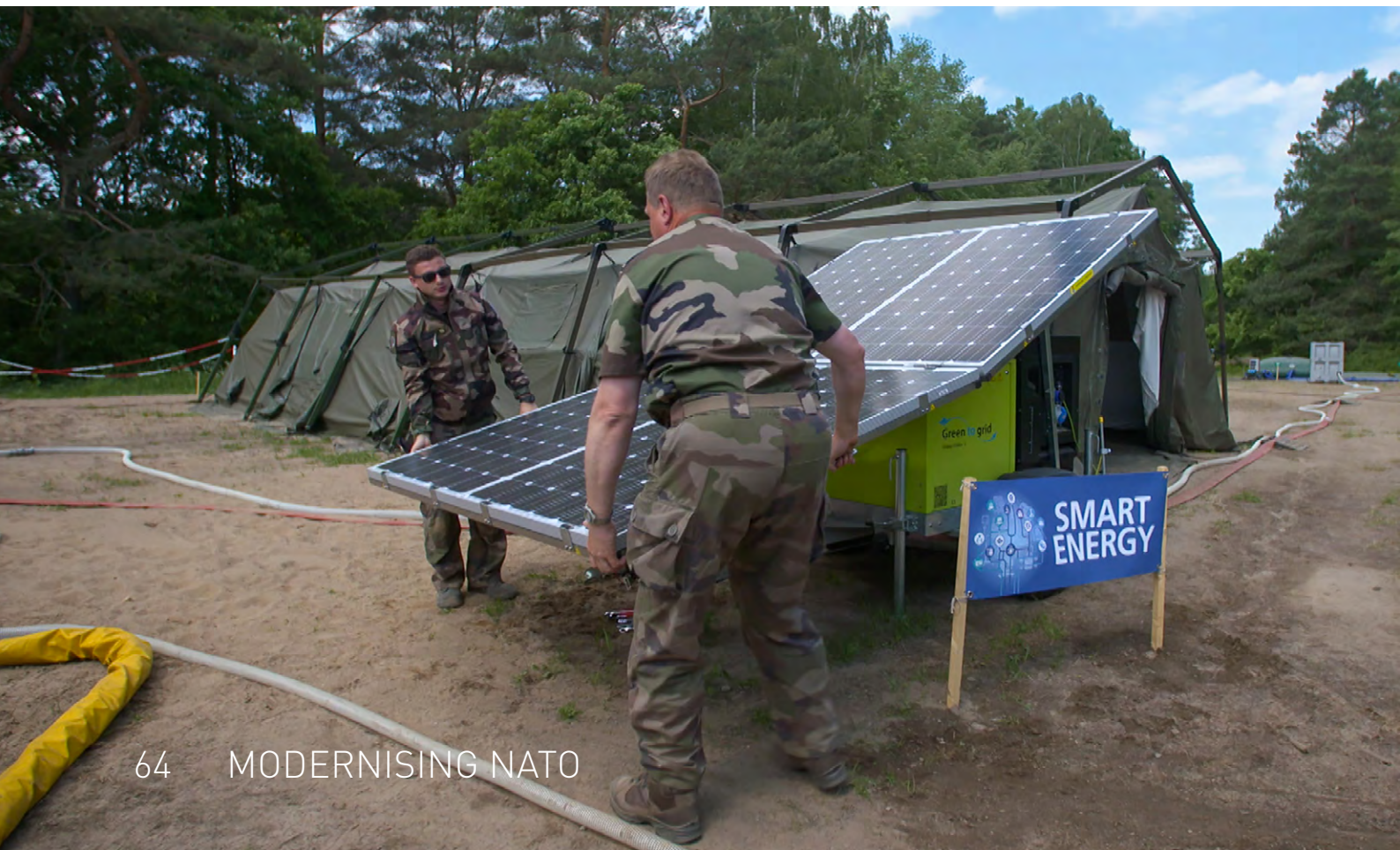
French Air Force personnel unfold photo-voltaic solar panels connected to a "green to grid" portable trailer during Exercise Capable Logistician 2019. Drawsko Pomorskie Training Area, Poland. June 2019.
